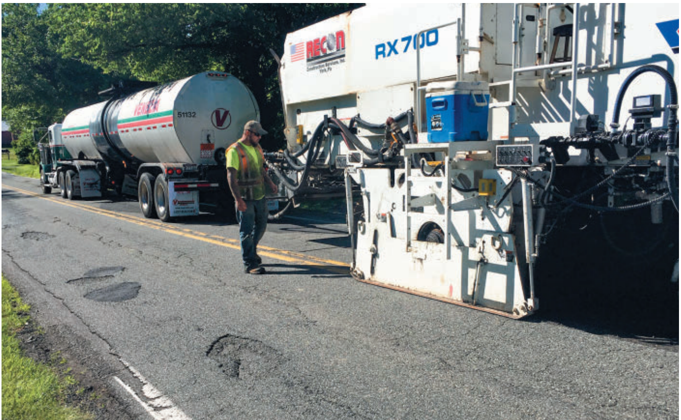
Roadtec RX-700 mill provides initial surface recycling with tanker supplying CSS-1h asphalt emulsion
